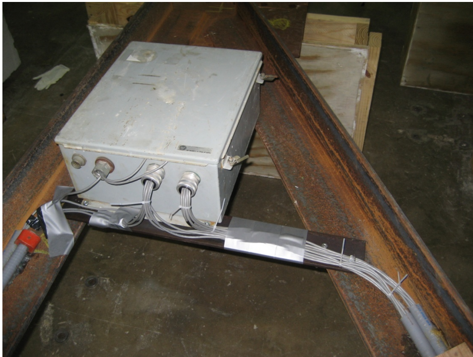
Figure 2.12 Multiplexer in Metal Box Mounted on Cross Frame
