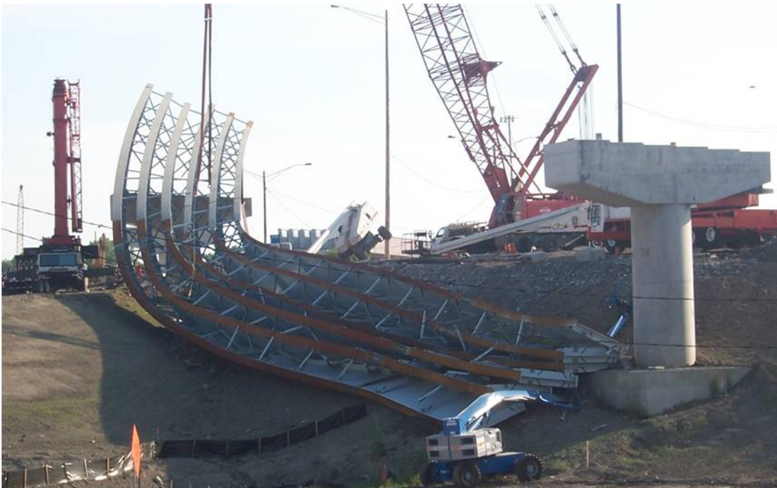
Figure 1.1 Curved Bridge Collapse
